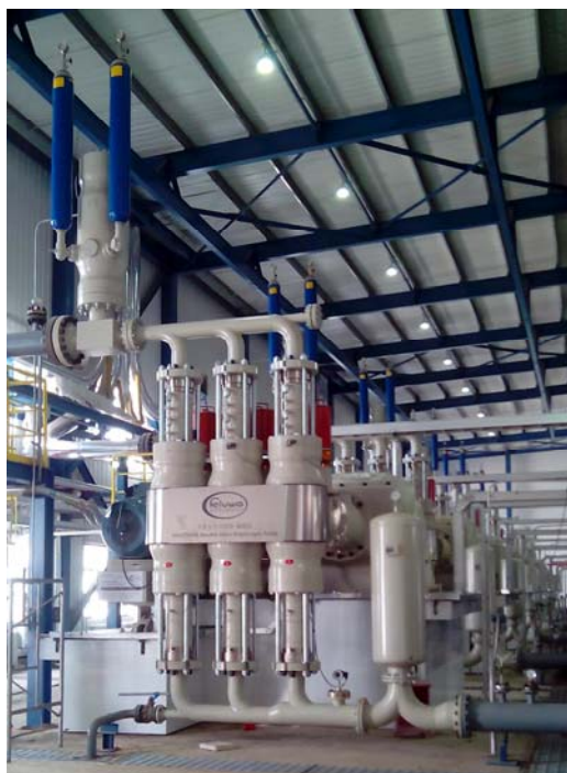
Figure 1. Seven sets of double hose-diaphragm pumps.
